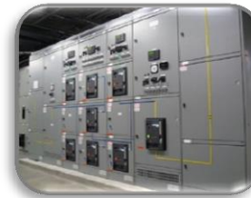
- Critical Meter Rooms
